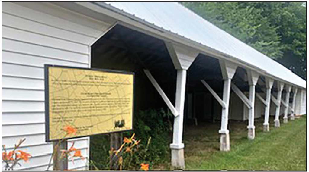
Jerusalem Church horse shed constructed in 1897 with modifications in 1914, 1932 and 1957. It is marked with a placard as part of Shawano County's "From the Pineries to the Present" project.
